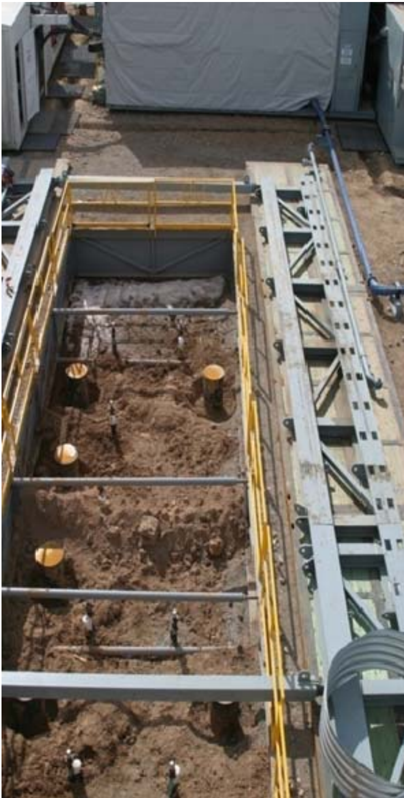
Figure 4. Cellar showing various conductor pipes for wells. Also shown is the rail system for moving the rig.
